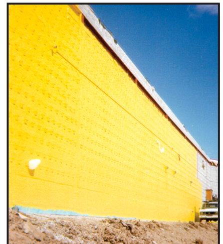
Above: Rub-R-Wall AVB applied over outer surface of inner wythe of masonry wall.
